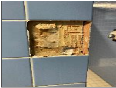
Non-asbestos yellow adhesive behind ceramic wall tiles in the Washrooms.
