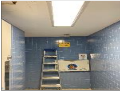
Drywall on the washroom ceiling.
