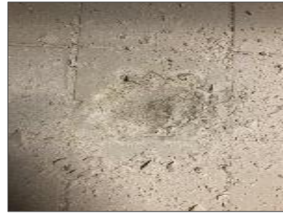
Non-asbestos thinset beneath in the Washrooms.
