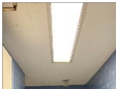
Flourescent lights in the Washrooms.
