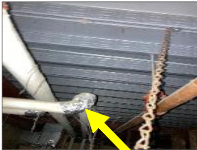
Pipes above ceiling are insulated with fibreglass and jacketed with paper and foil tape.
