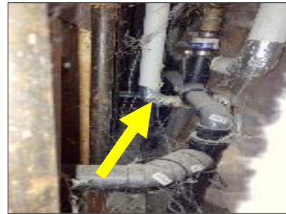
Pipes in pipe chase are insulated with fibreglass and jacketed with paper and foil tape.
