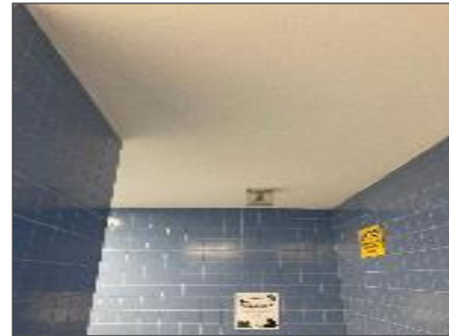
Emergency lighting in the Washrooms.
