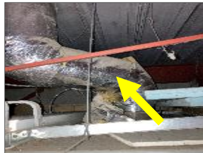
Ducts above the ceiling are insulated with fibreglass and jacketed with foil.
